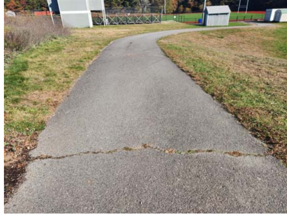
Figure 14 – Sample transverse pavement crack.
