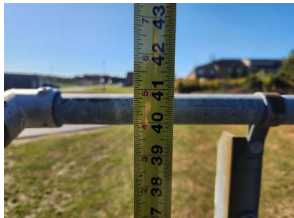
Figure 6 – Bleacher structure fall protection railing measured to be 41-inches from top of the timber seat.
