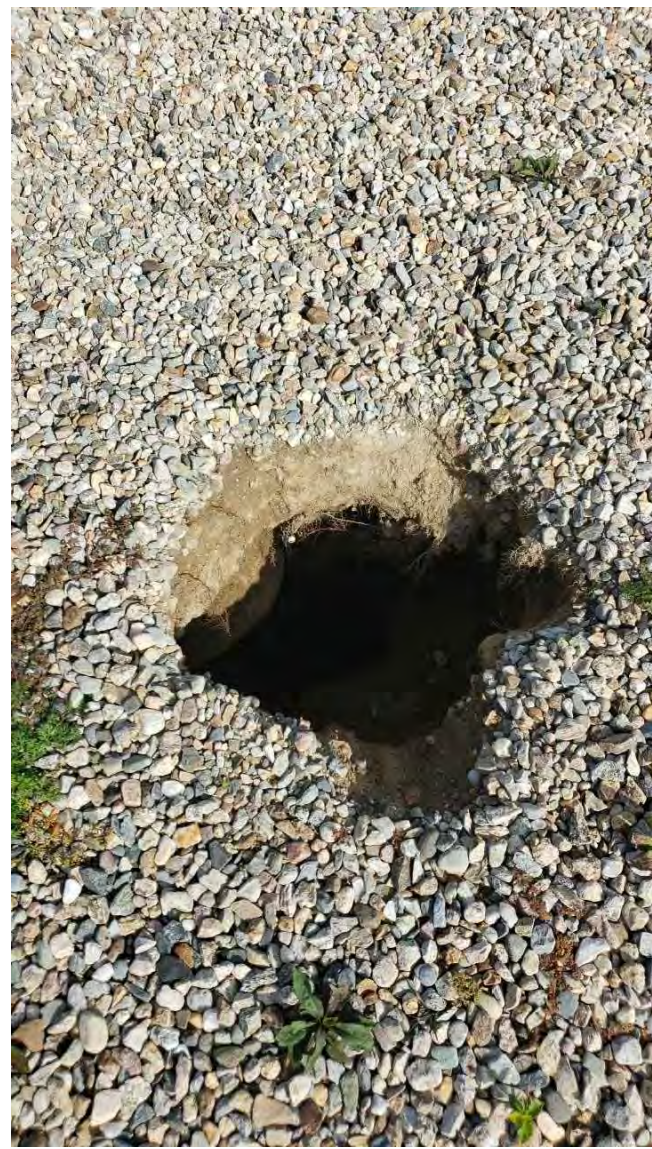
SINK HOLE IN GRAVEL SURFACE
