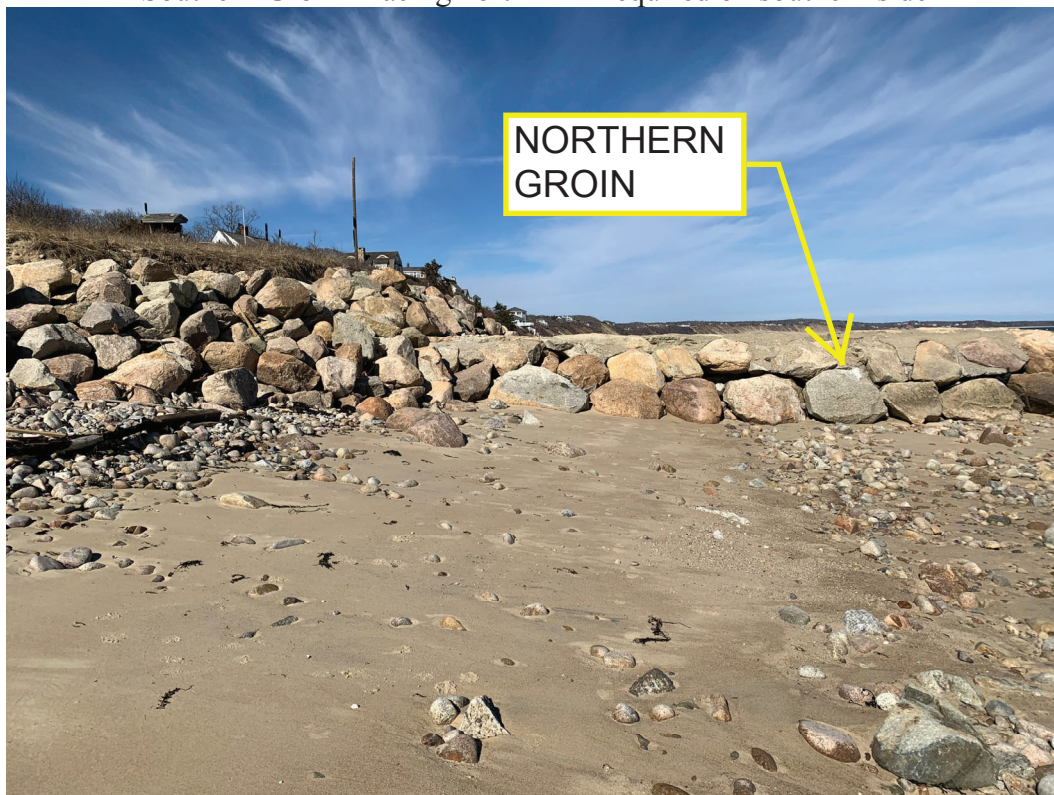
Northern Groin – facing north – fill required on southern side
