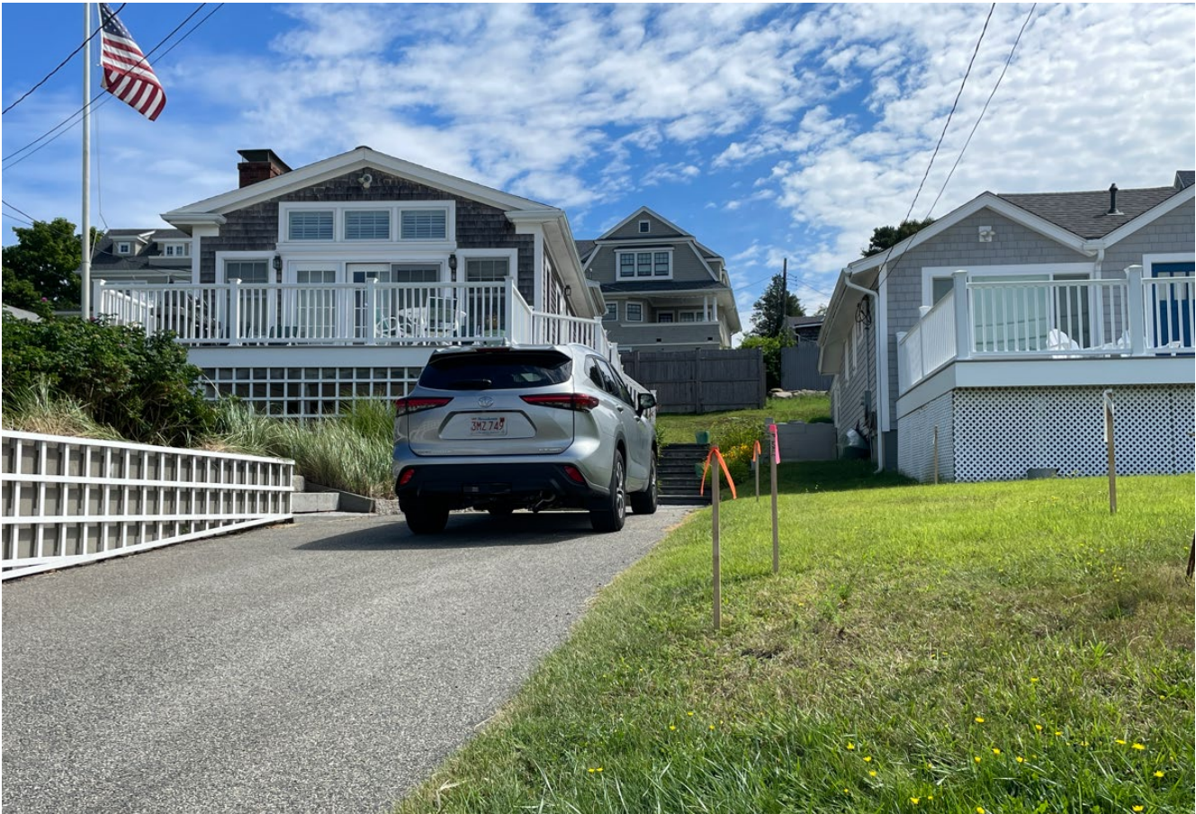
Photograph of Abutters Paved Driveway & limit of work and wall wooden bean posts
