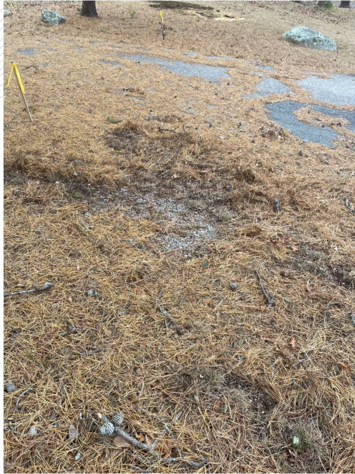
Picture 3 – view of the bank to the right of the yellow flag stakes, with pine needles removed by hand to expose existing peastone and pavement bank stabilization – no vegetation aside from one tree in this view.
