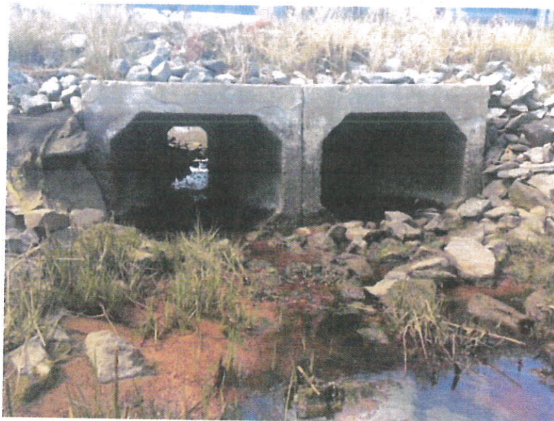
Figure 5: View of the culvert underneath Wings Neck Road. Facing north towards the marsh
