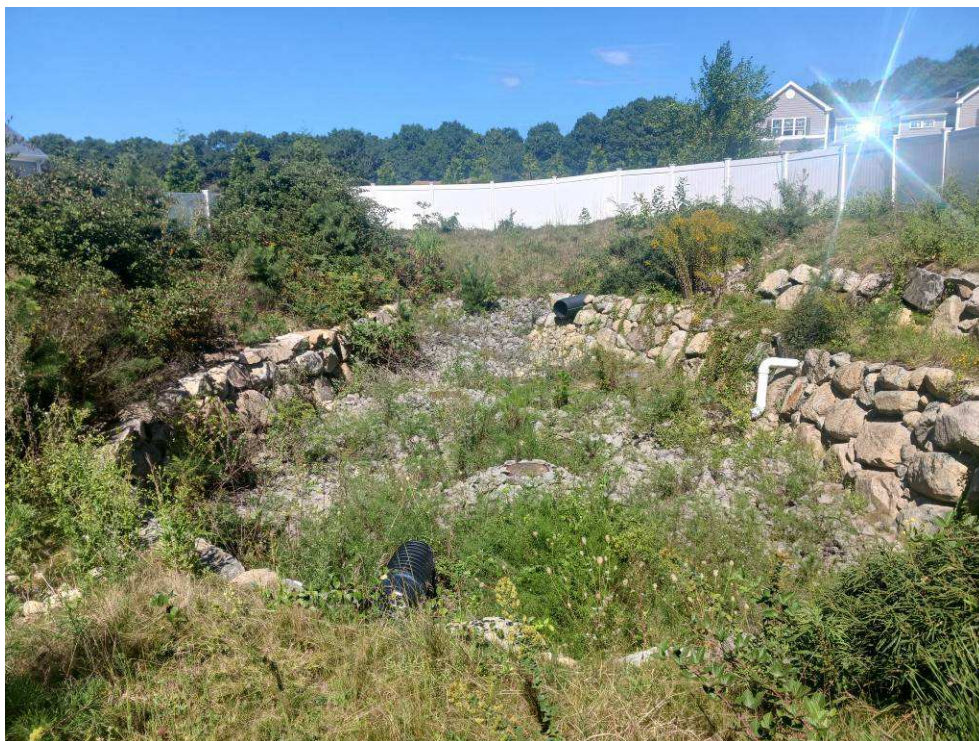
Figure 8 – Infiltration Basin Inlet (dry)
