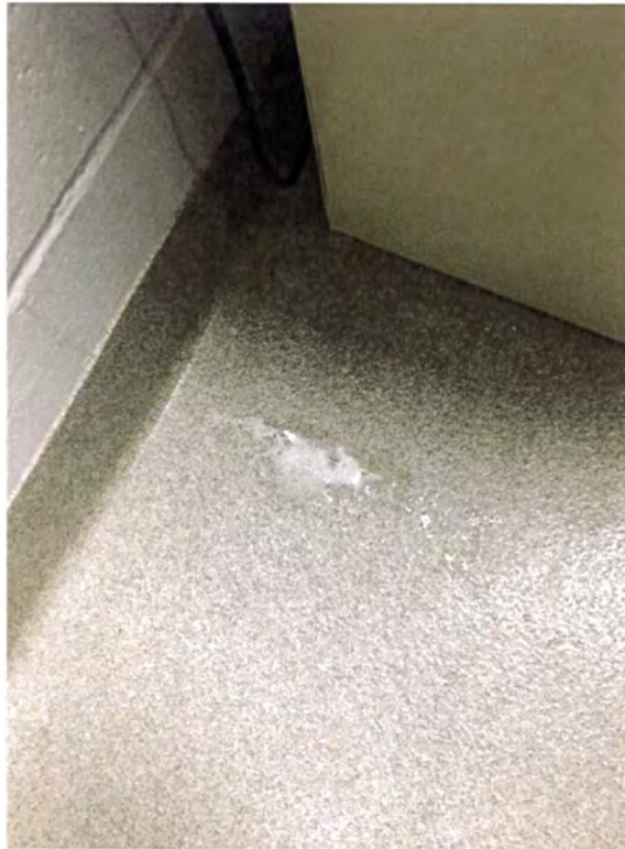
Photograph 9 Water leakage on interior of Kitchen Office 153
