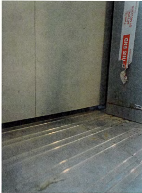
Photograph 11 Daylight visible at closure joint of Gymnasium Door
