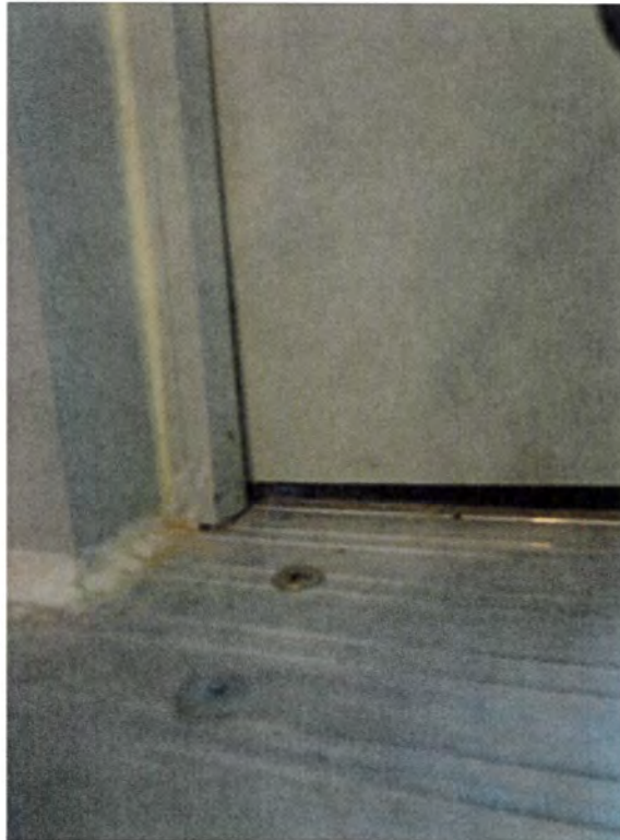
Photograph 12 Daylight visible at hinge of Gymnasium Door
