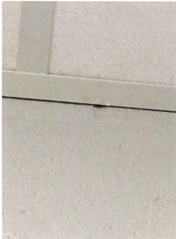
Photograph 10 Water leakage on interior of Kitchen Office 153
