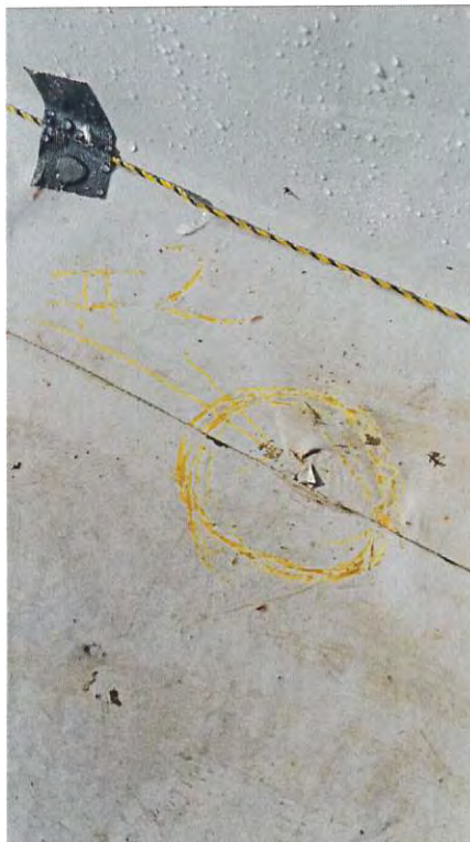
Photograph 10 Void in field-welded seam at parapet by monitor wall above second floor classroom
