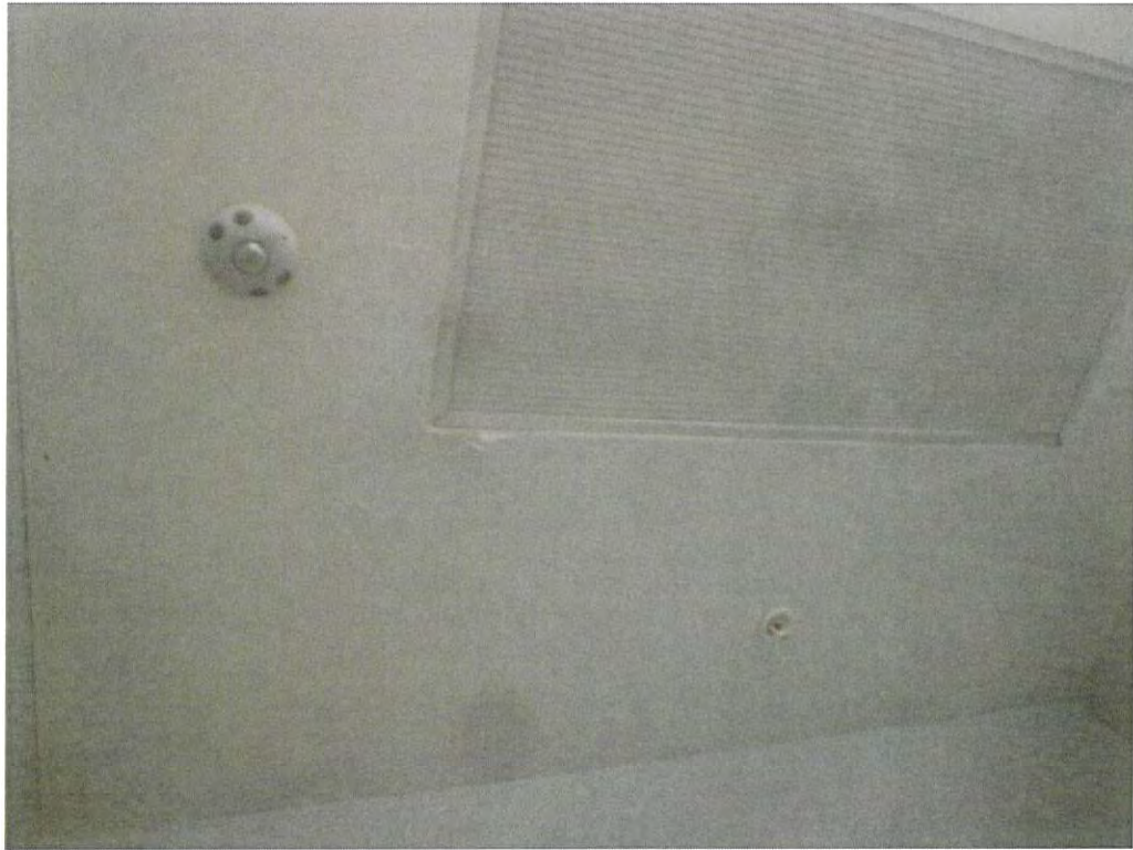
Photograph 29 Blistered paint on ceiling by Bathroom Area duct vent
