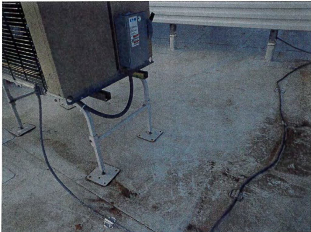
Photograph 30 Metal feet of equipment frames set directly on Sarnafil membrane
